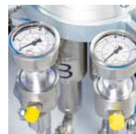
Pressure gauge units at machine outlet for component A and component B
